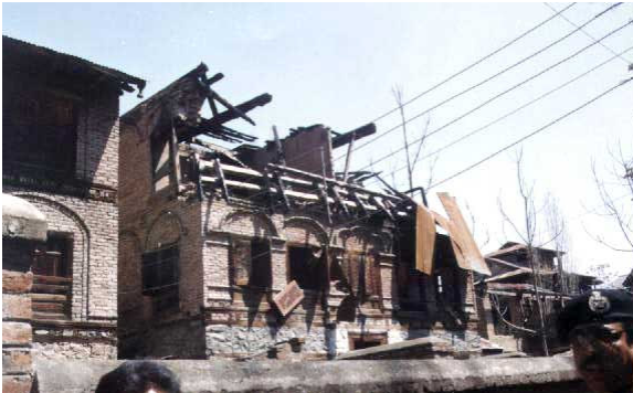
The ugly face of terrorism: Destroyed homes of community
